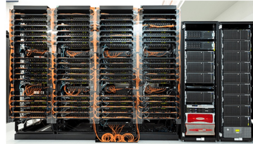
MDGRAPE-4A Full System: 64 Boards
